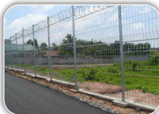
Pagar Wire Mesh Wire Mesh Fence
