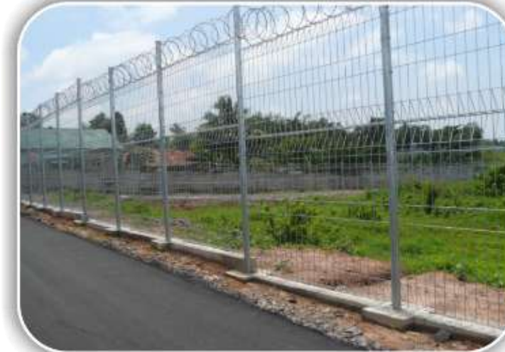
Pagar Wire Mesh Wire Mesh Fence
